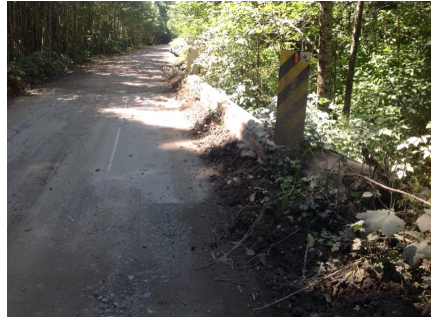
sediment on deck against guardrail
